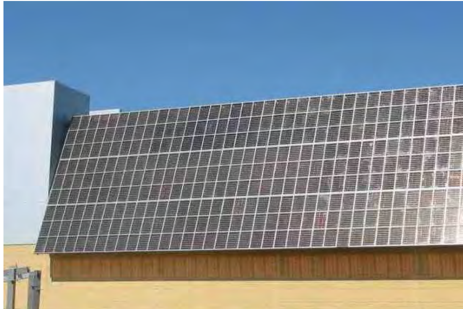
DSSC Façade System at the CSIRO Energy Centre Newcastle, Australia
